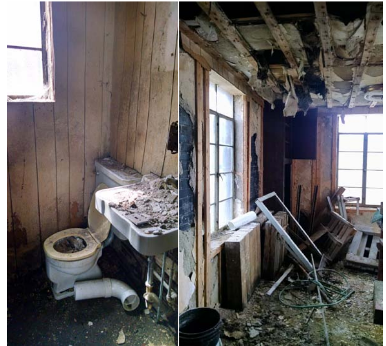
Inside powerhouse, bathroom and office showing significant damage. Existing
