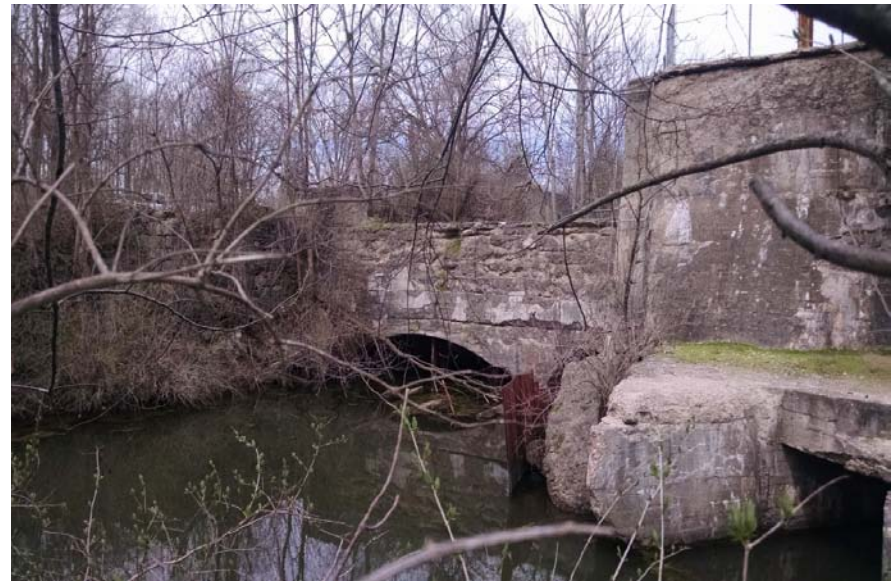
Looking upstream at abandoned spillway/old foundation of 1897 powerhouse (old powerhouse foundation pictured below). Existing
