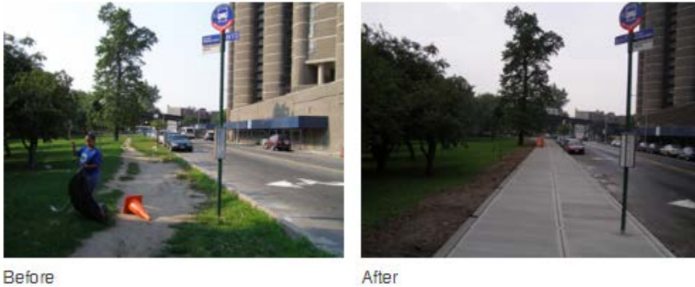
Figure 9 Bus Stop at Mosholu Parkway and Paul Avenue in the Bronx, NY
